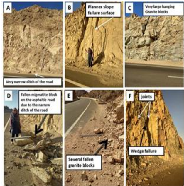
Fig.13: Different sites of slope instability hazards along Sohag-Red Sea asphaltic roads. (A) a very narrow and flat ditch of the road(B) and (F) show planner and wedge slope failure. (C) a very large unstable hanging granite blocks.(D) and (E) show different sizes of fallen basement blocks on the asphaltic road.
